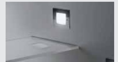
Modular LED stairlight fitted into a Define® New Media™ plate
